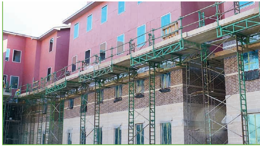
Guardrails are installed on the ground and stay in place as the wall is built. No one ever leaves the "safety zone" on adjustable scaffolding.
