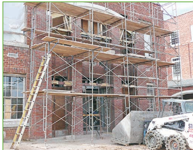
Photo 4: Providing safe access to conventional scaffolding can be tricky. This extension ladder only provides access to the first level. Clamp-on ladders might be better here.
