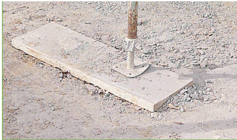
Photo 1: Short mud sills reduce shovel work and insure that they won't be re-used for scaffold planks.
