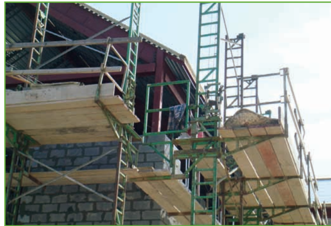
Photo 3: Guardrails, end rails, and safe access are always in place on crank-up style scaffolding. The towers are legal to climb.
