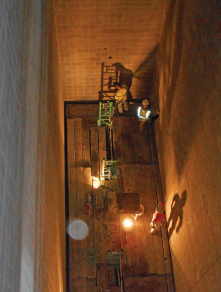
Photo 2 - The walls were rubbed down as the scaffold was lowered down to the basement.
