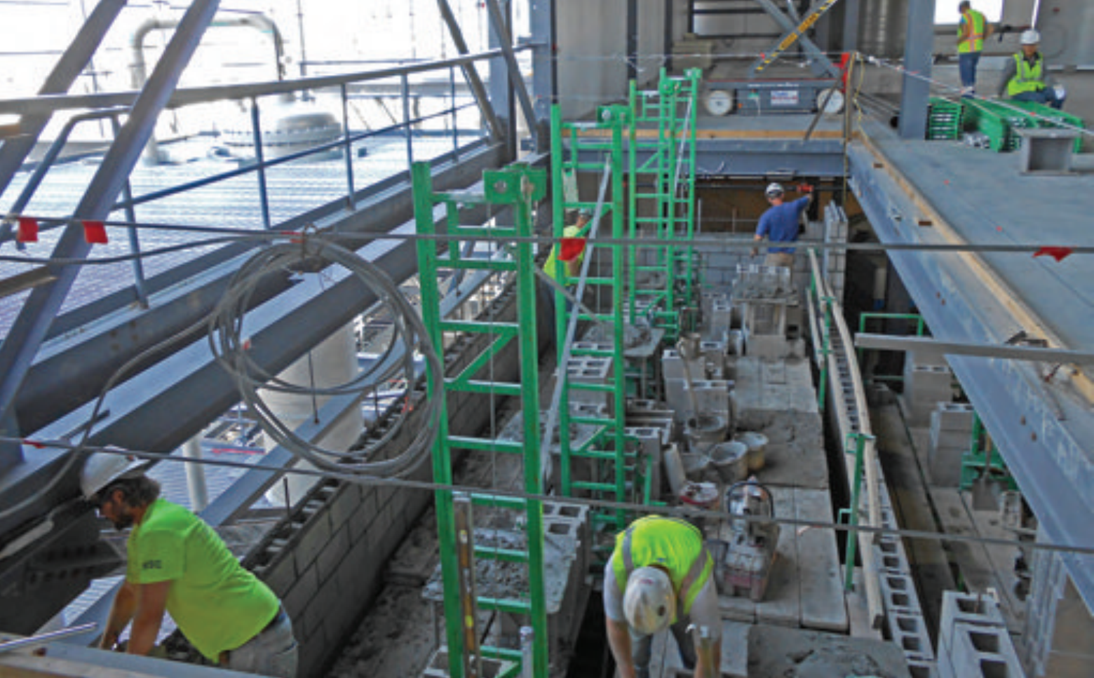
Photo 1 - Seedorff Masonry used Non-Stop scaffolding in a 90-foot-high elevator shaft. The masons outriggers and Inside Corner Arms were used to fully plank the inside of the shaft.
